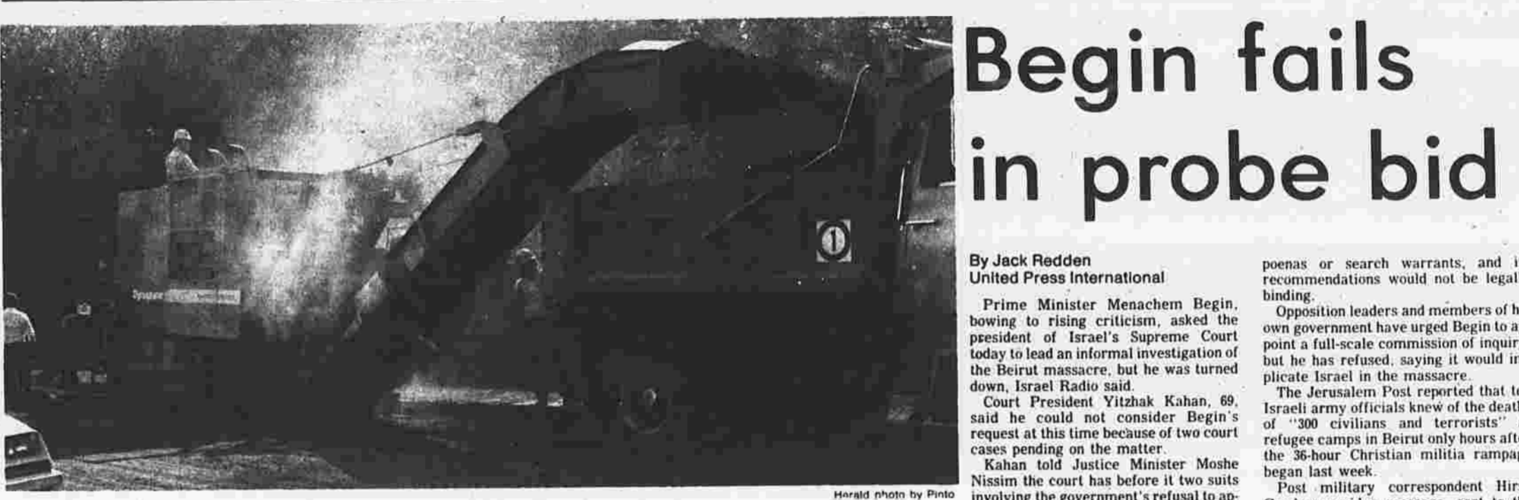
Workers are picking up the surface of Main Street and putting in the trucks where it will bounce no more drives and break no more shocks. When the old surface is carved off, a new one will be put on and the driving will be smooth again from the Center to Hillard Street.
